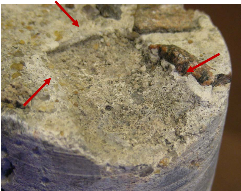
Figure 4. Depression left when relatively large coarse aggregate particle separated from top surface, arrows indicate original outline of particle. For scale, the width of the socket is approximately 1 inch.
