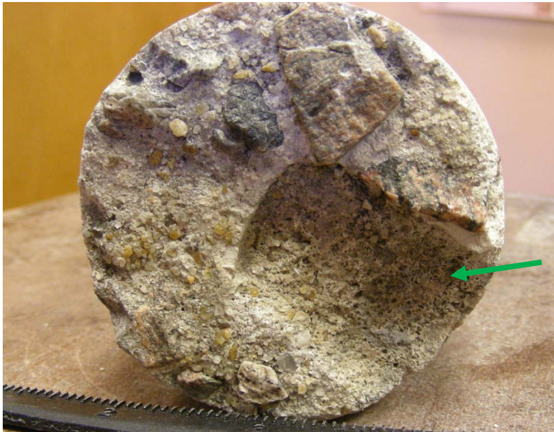
Figure 2. Top surface of core, representing significantly deteriorated top surface of apron. A large coarse aggregate particle (socket is 1-1/4 in. long and 1 inch wide) is indicated by the arrow.
