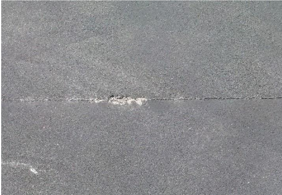
Photograph 33: Typical Transverse Cracking (medium-severity)
