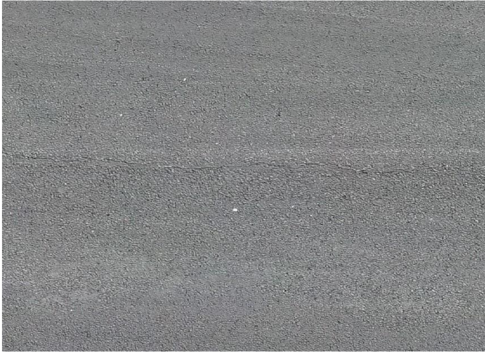
Photograph 35: Typical Longitudinal Cracking (low-severity)
