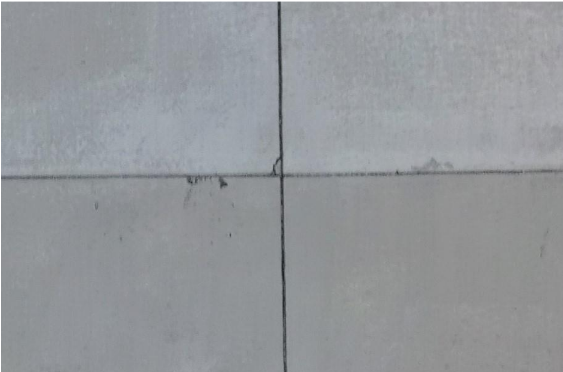
Photograph 2: Typical Joint Spall (low-severity) and Corner Spall (low-severity)
