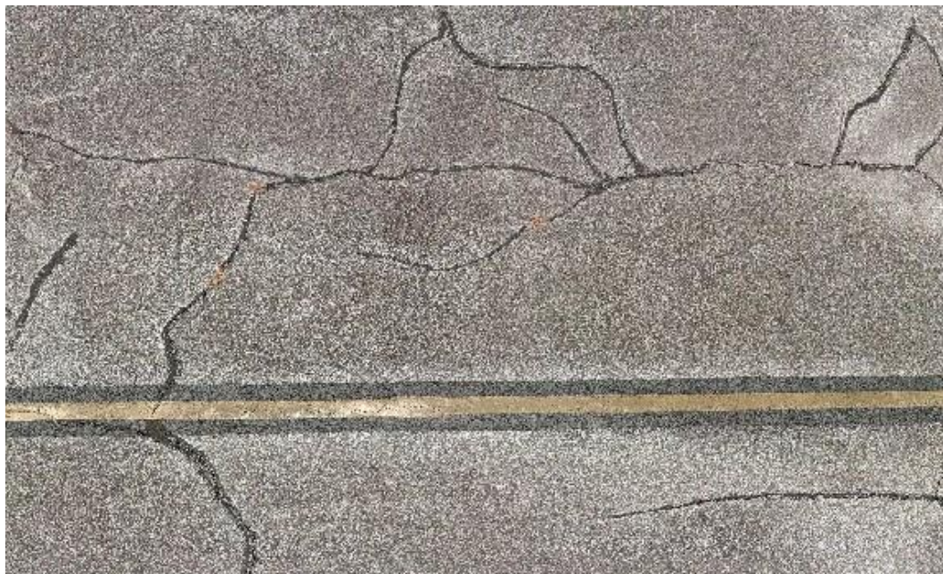
Photograph 12: Alligator Cracking (Low-Severity) and Weather (Low-Severity)
