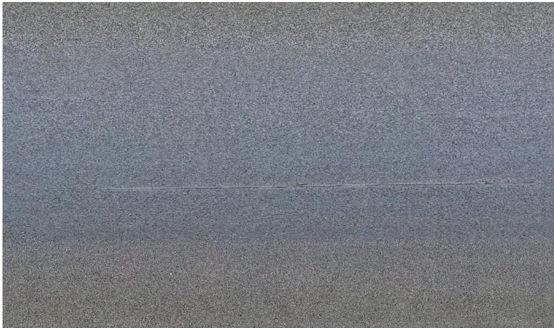
Photograph 30: Typical Longitudinal Cracking (low-severity)
