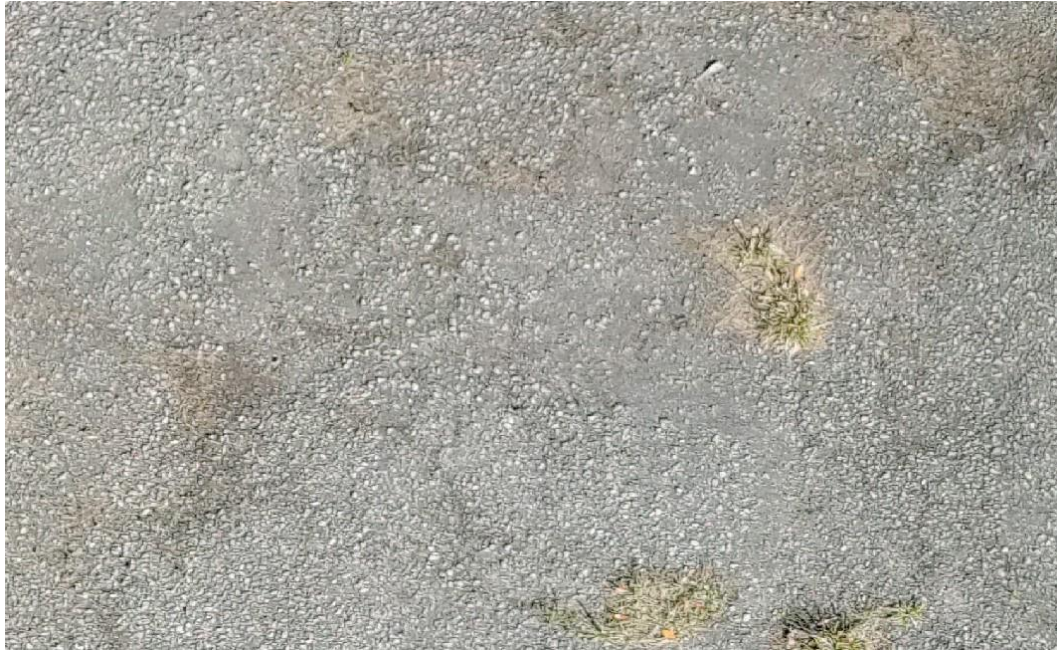
Photograph 17: Alligator Cracking (Medium-Severity)
