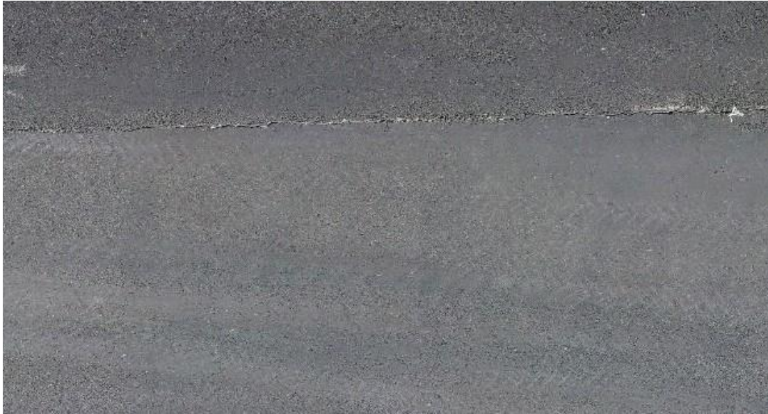
Photograph 29: Typical Longitudinal Cracking (medium-severity)
