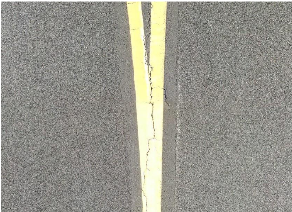
Photograph 46: Typical Longitudinal Cracking (low and medium-severity)
