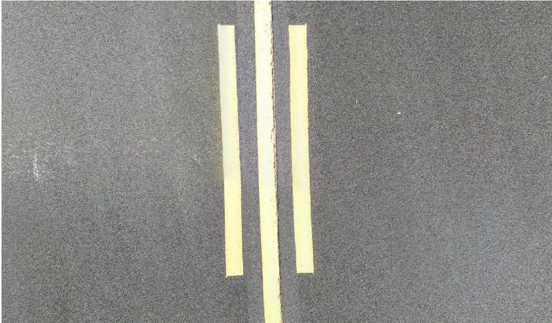
Photograph 49: Typical Longitudinal Cracking (medium-severity)
