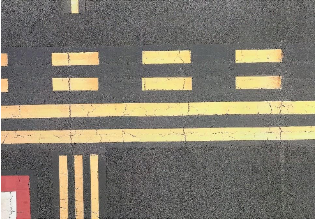
Photograph 37: Typical Longitudinal Cracking (medium-severity)
