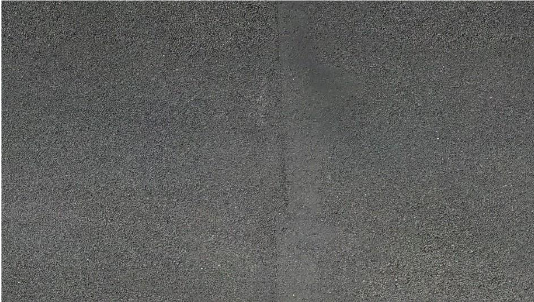
Photograph 23: Typical Transverse Cracking (medium-severity)
