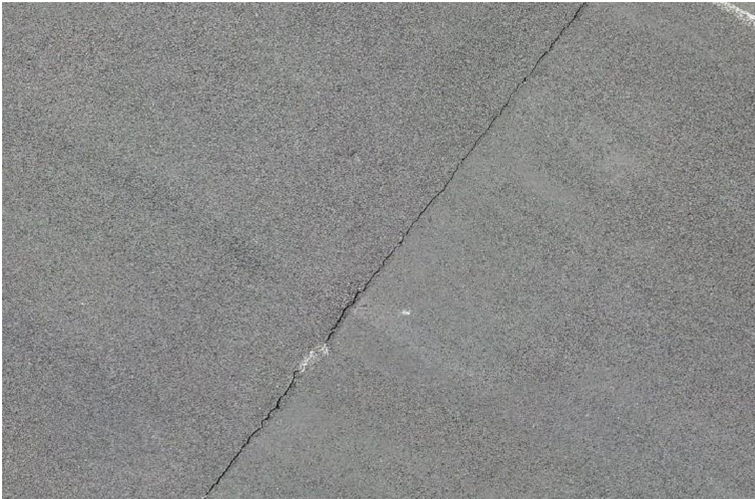
Photograph 50: Typical Transverse Cracking (medium-severity)
