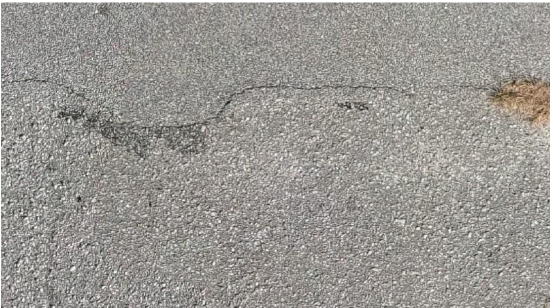
Photograph 26: Typical Transverse Cracking (low-severity)
