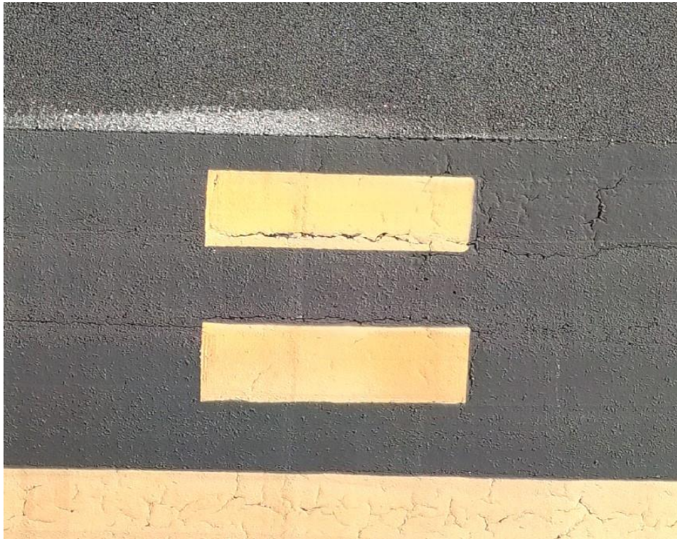
Photograph 45: Typical Longitudinal Cracking (medium-severity)
