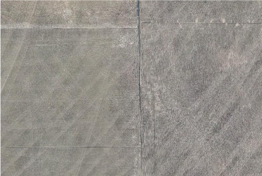
Photograph 3: Typical Linear Crack (low-severity)
