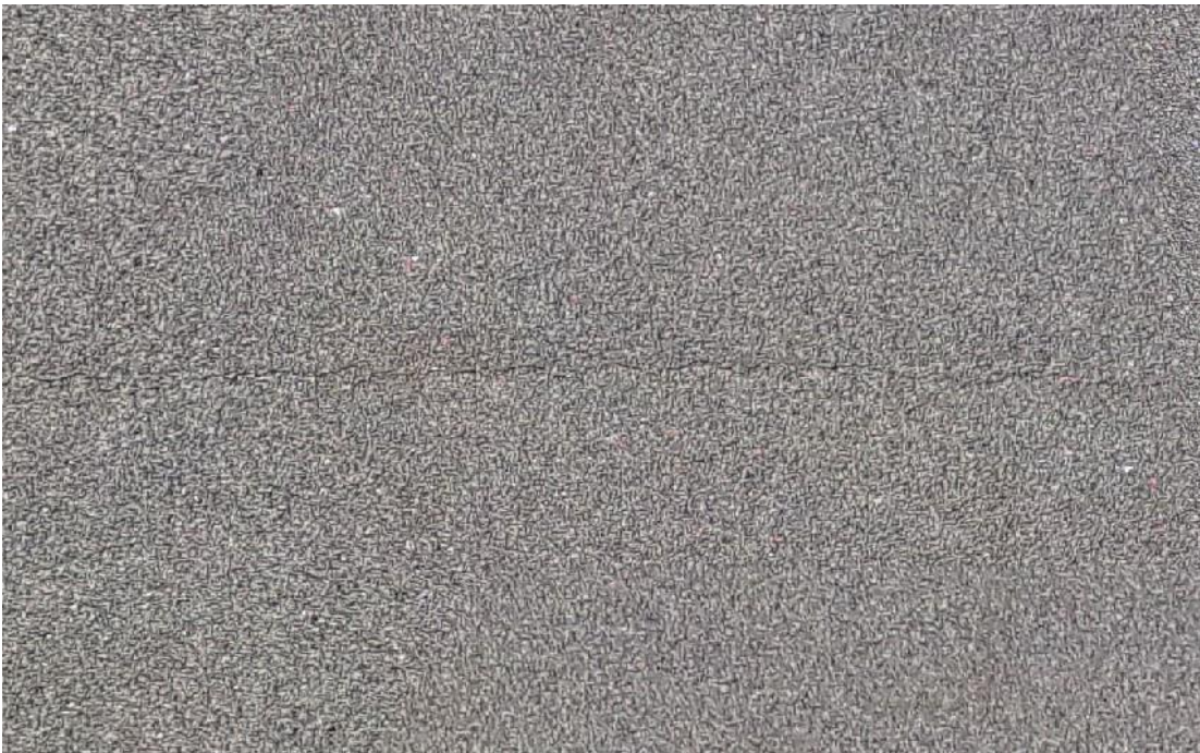
Photograph 14: Typical Longitudinal Cracking (Low-Severity) and Weathering (Low-Severity)
