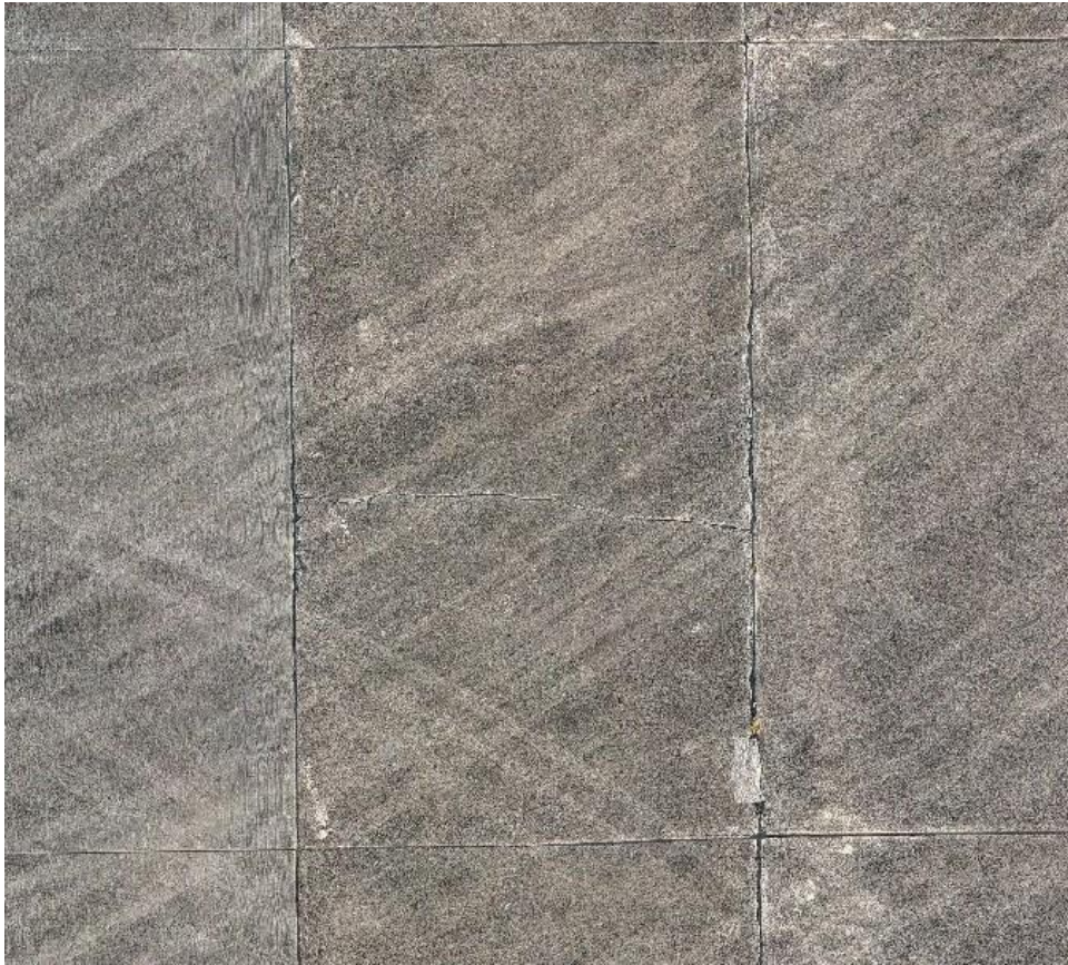
Photograph 43: Typical Linear Crack (medium-severity)
