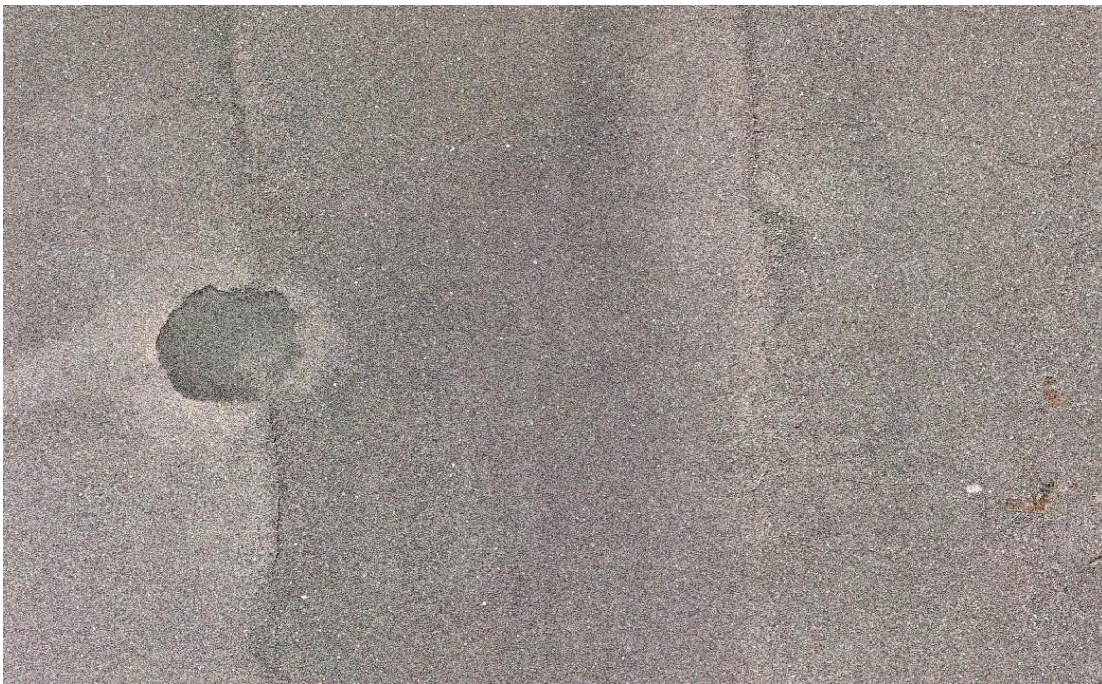
Photograph 10: Patching (Low-Severity) and Longitudinal and Transverse Cracking (Low and Medium-Severity)
