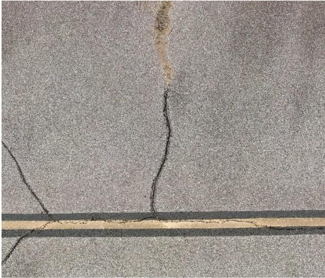
Photograph 11: Typical Longitudinal and Transverse Cracking (Medium-Severity)
