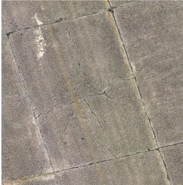
Photograph 5: Shattered Slab (high-severity)
