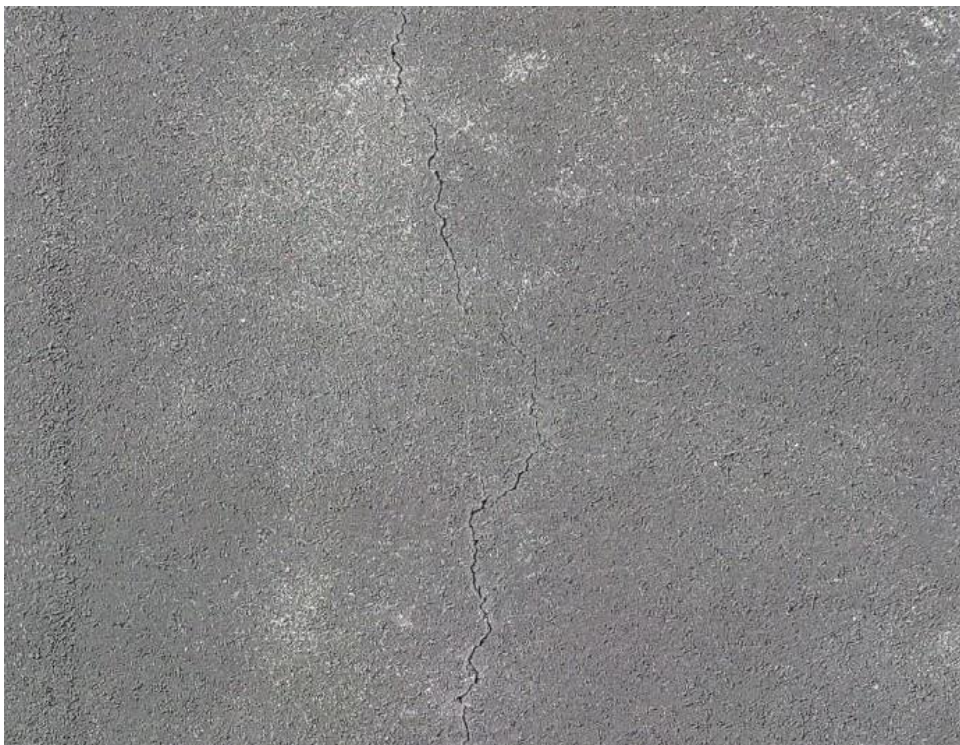
Photograph 16: Typical Longitudinal Cracking (Low-Severity) and Weathering (Low-Severity)
