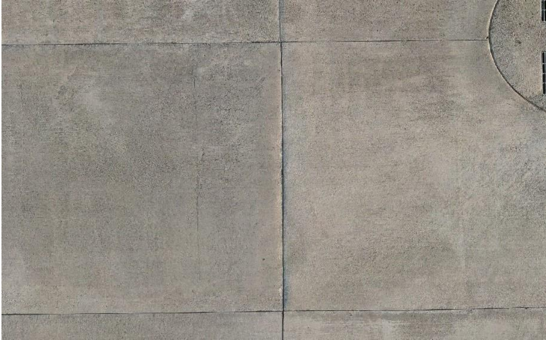
Photograph 1: Typical Linear Crack (low-severity)
