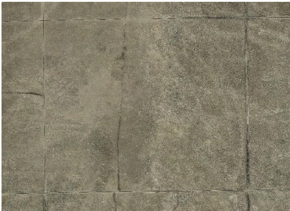
Photograph 8: Typical Linear Crack (medium-severity)
