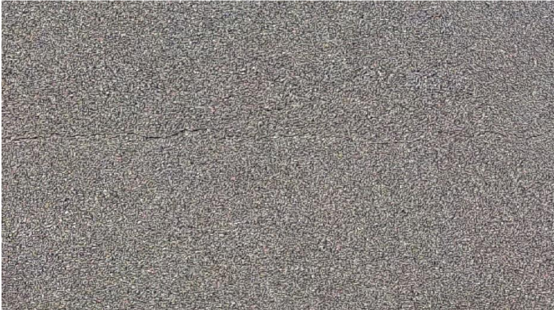
Photograph 13: Typical Longitudinal Cracking (Low-Severity) and Weathering (Low-Severity)
