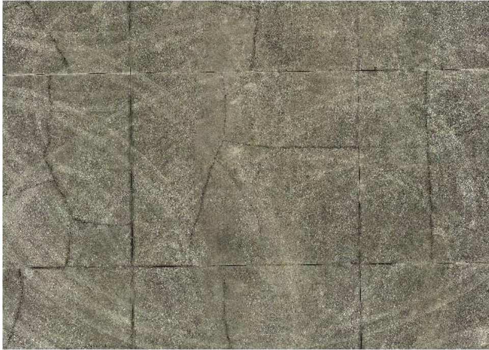
Photograph 7: Typical Shattered Slab (medium-severity)
