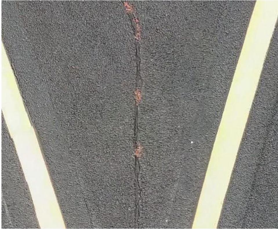
Photograph 47: Typical Longitudinal Cracking (medium-severity)
