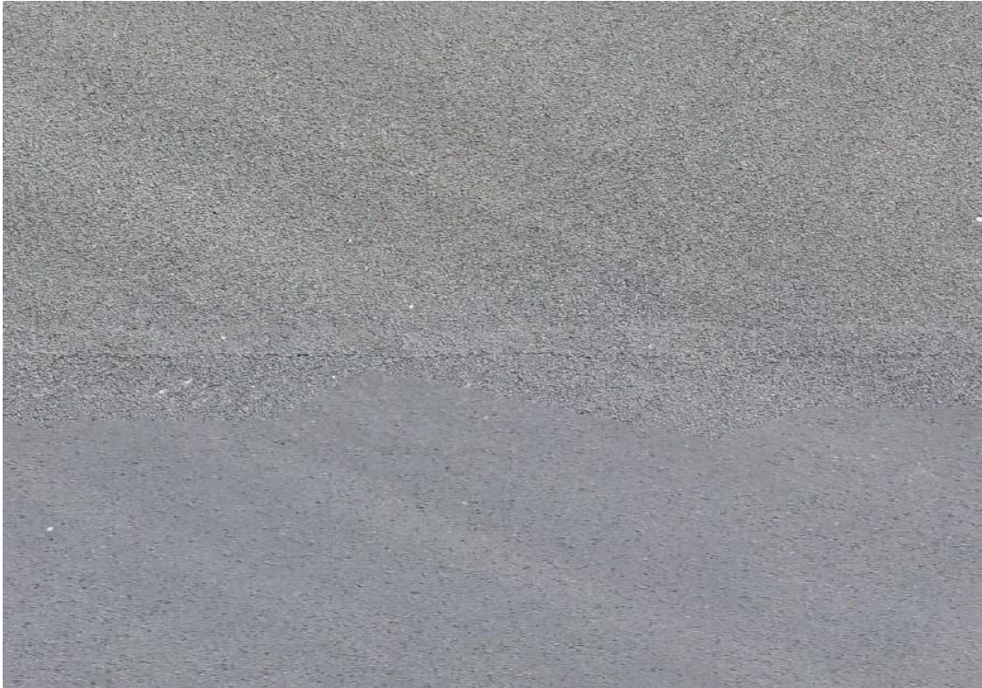
Photograph 39: Typical Longitudinal Cracking (low-severity)
