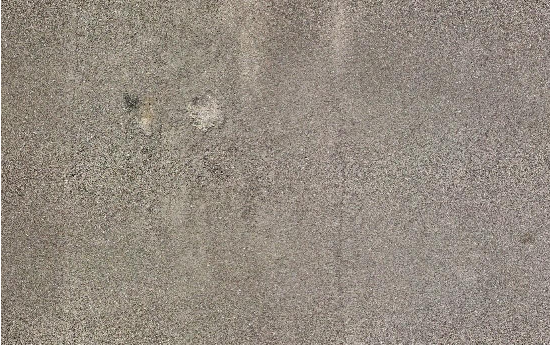
Photograph 9: Alligator Cracking (Low-Severity)
