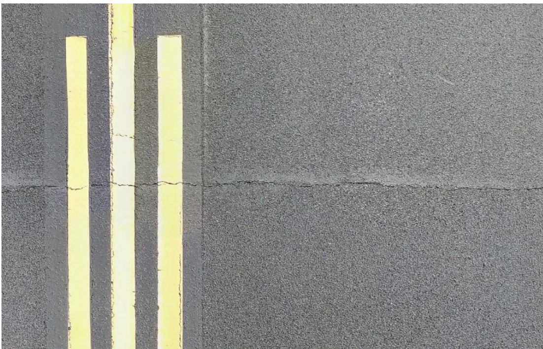
Photograph 40: Typical Longitudinal Cracking (low-severity)
