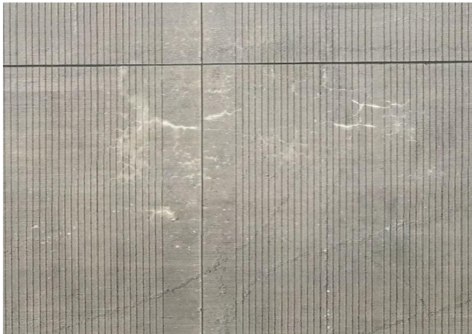
Photograph 22: Typical Shrinkage Cracking (low-severity)
