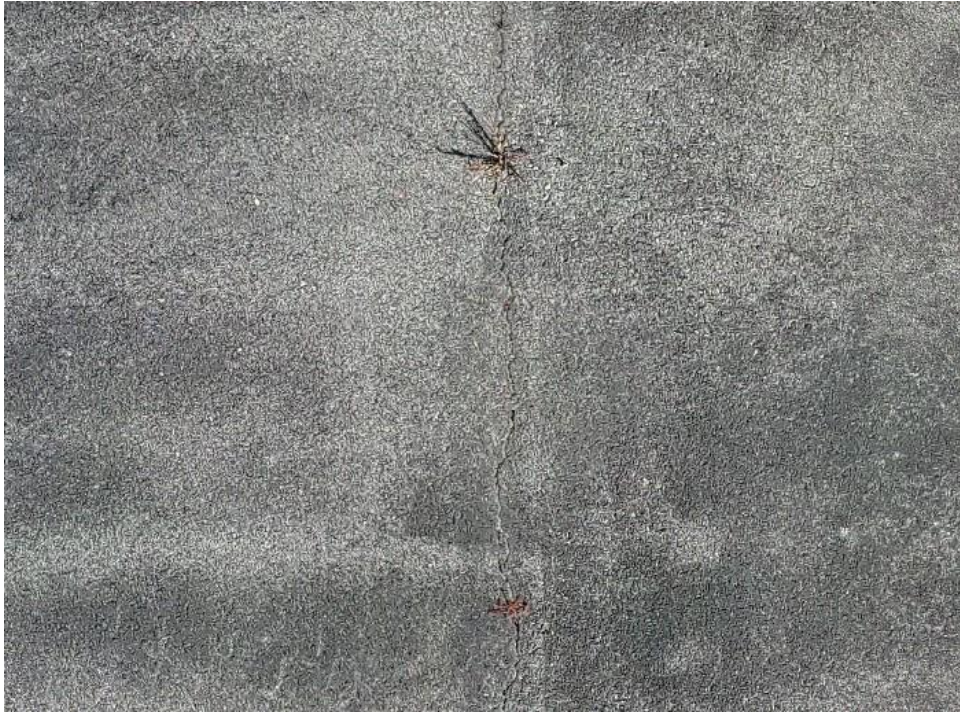
Photograph 15: Typical Longitudinal Cracking (Medium-Severity) and Weathering (Low-Severity)
