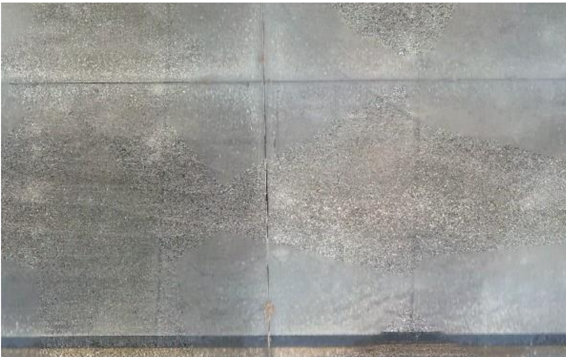
Photograph 4: Typical Joint Sealant Damage (low-severity)
