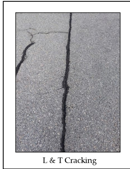
Figure I.12: Examples of Distresses on Taxiway B System, CAE
