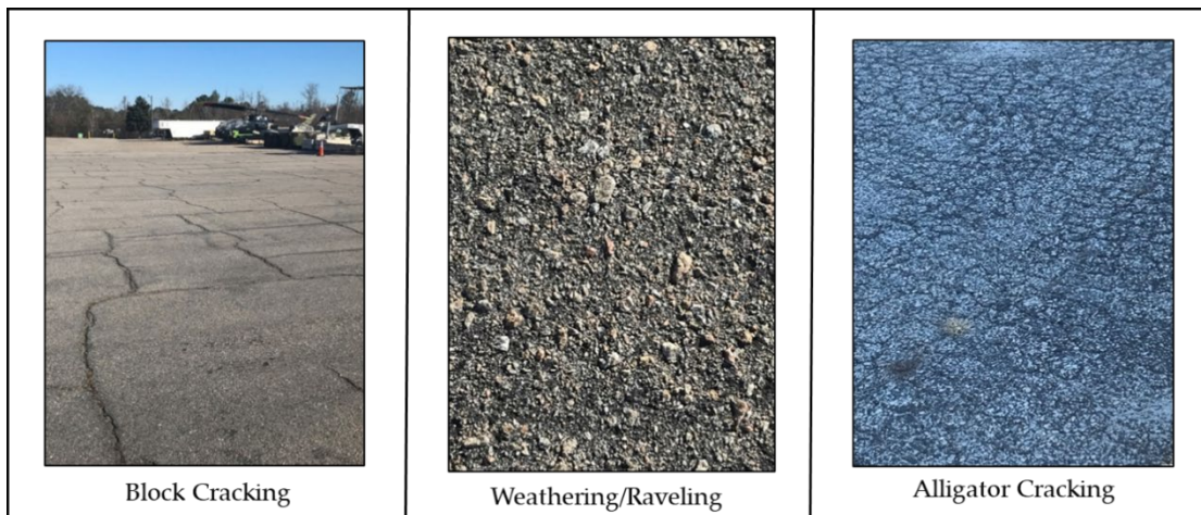
Figure I.17: Examples of Distresses on Taxiway S, CAE
