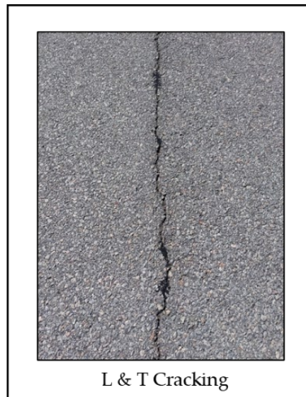
Figure I.14: Examples of Distresses on Taxiway D System, CAE
