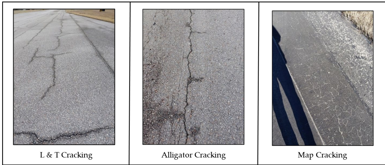
Figure I.13: Examples of Distresses on Taxiway C System, CAE
